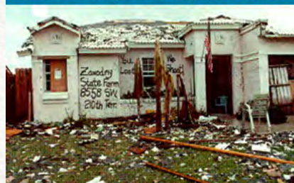
Level 3 - Major damage; uninhabitable
